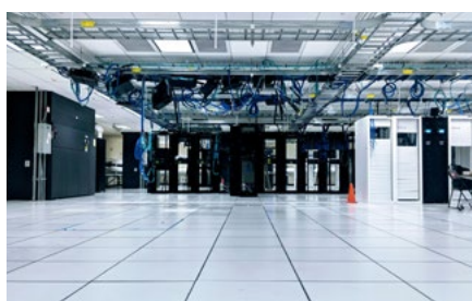
Data centres and telecoms
